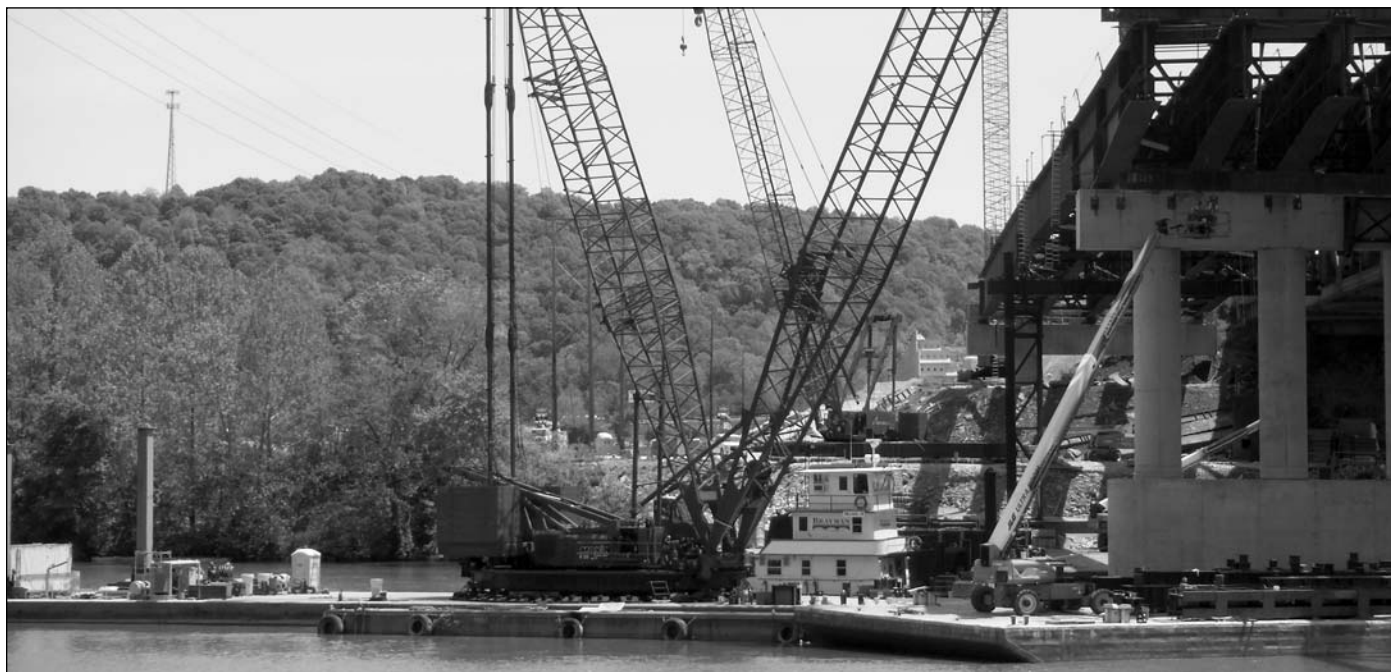
The construction of the Nitro-St. Albans bridge on I-64 west of Charleston, West Virginia. Projects like this one were analyzed throughout Kentucky for the recent study on prevailing wage, which determined there had been no cost savings to the state since the repeal of the law.
