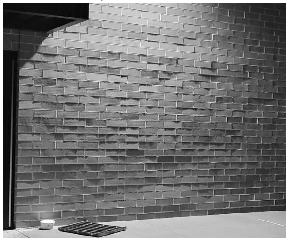
Brick work rejected at Monroe school project which GC DCI/Shires claims is fine.
