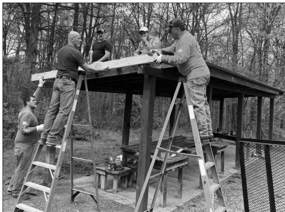
(From left) SMART Local 33 members John Young, Jim Jackson, Jeff Fry, Chris Garrett and Steve Perdue volunteer to replace a roof at the public shooting range in the Pleasant Creek Wildlife Management Area.
