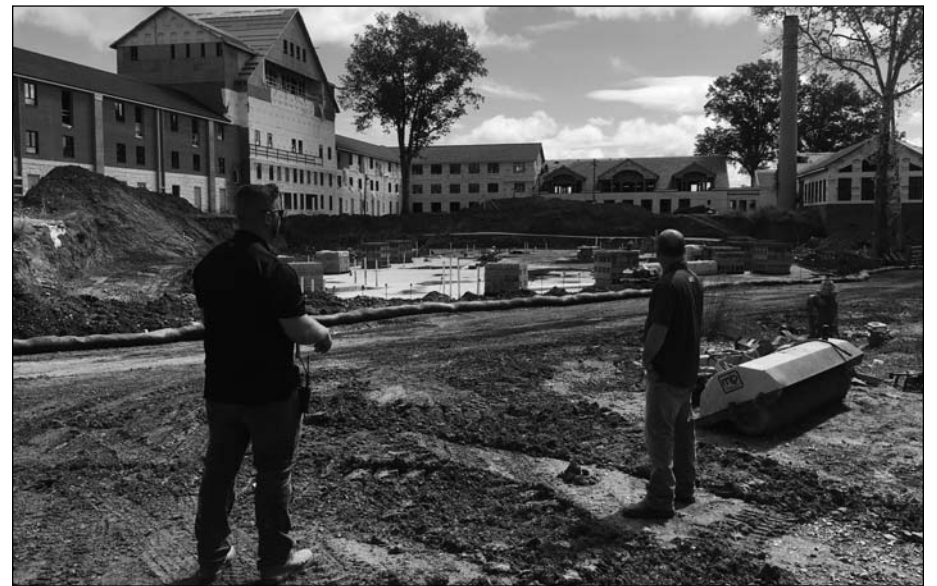
Steve Matheny (left) of Matheny & Sons General Contractors talks with Randall May of the Carpenters in front of the new 108 room resort called The Grand Patrician in Milton.
