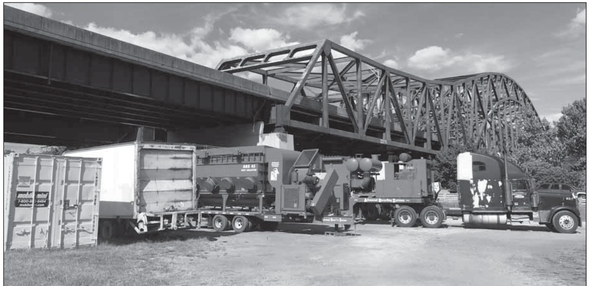
The Chuck Yeager Bridge in Kanawha County is being painted by Florida based International Rigging Group, a company which is owned by the same people who just plead guilty to fraud on a similar project being done in West Virginia under a different company name. The company is not in compliance with the West Virginia Jobs Act which requires local hiring for tax funded projects.
