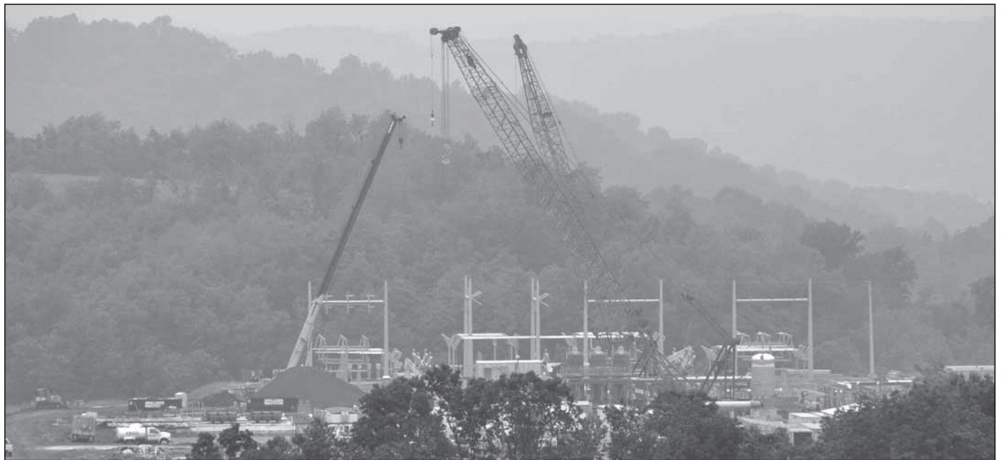
Williams Partners has hired union contractor URS to build this natural gas processing facility at Oak Grove, in the Wheeling area. This project employs hundreds of local union construction workers and is one of several natural gas processing facilities under construction to meet the needs of Marcellus and Utica Shale gas.
