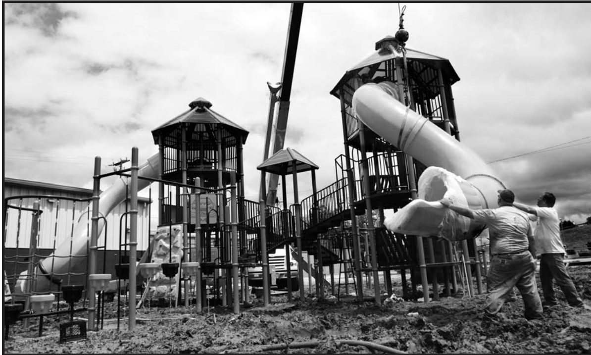
VOLUNTEERS A. JAY BOOTH, IBEW 317 (left) and Roger Johnson, Carpenters 1207 guide a slide into place at the Kellogg Elementary School playground. The crane was on loan from Neighborgall Construction. Photo courtesy of the The Herald-Dispatch, Huntington, W.Va.
