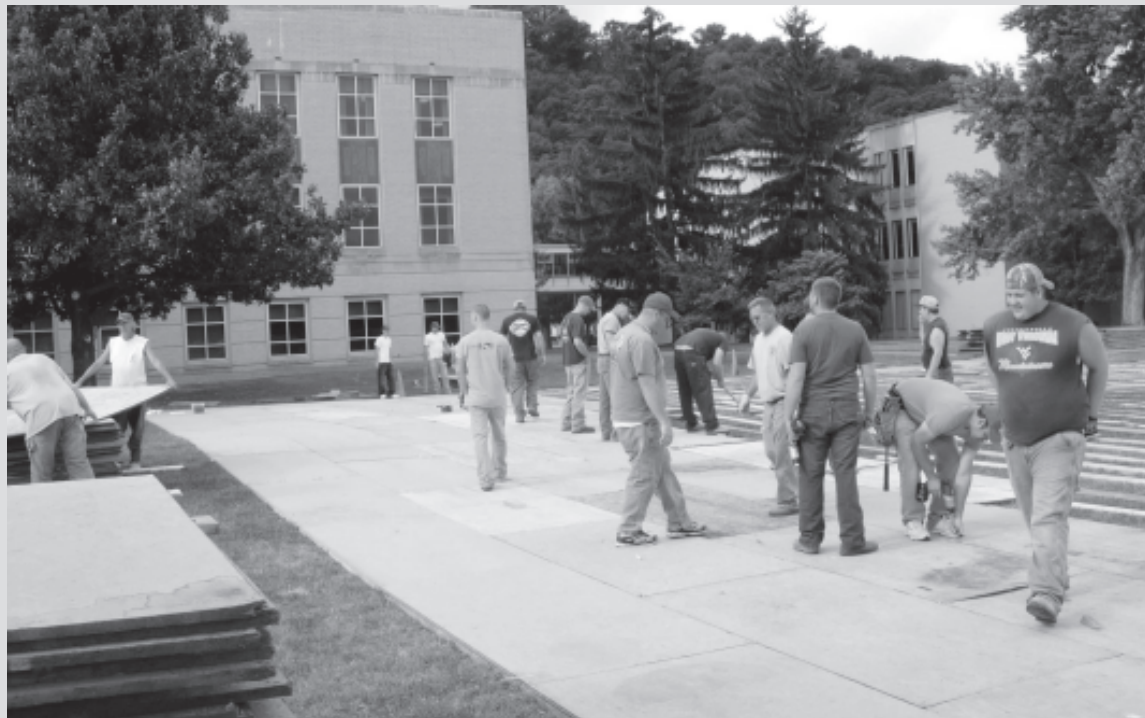
APPRENTICES AND JOURNEYMEN from Carpenters Local 302 and 1207 as well as Laborers Local 1353 helped install a dance floor for a local charitable event. The 220 by 80 foot floor was used for a September 19 fundraiser called "Starry Starry Night," to raise money for a new, $20 million athletic complex at the University of Charleston. Actress Jennifer Garner and her husband Ben Affleck attended. Local contractors BBL Carlton and Cornerstone Interiors also helped in the effort.
