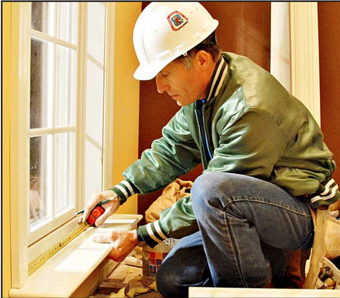
MIKE BRUFFEY, A member of Carpenters Local 476, Clarksburg, installs trim at the Extreme Makeover home in Fairmont. Bruffey, a second generation carpenter from Weston, joined with other volunteers to make the week long project a success.
